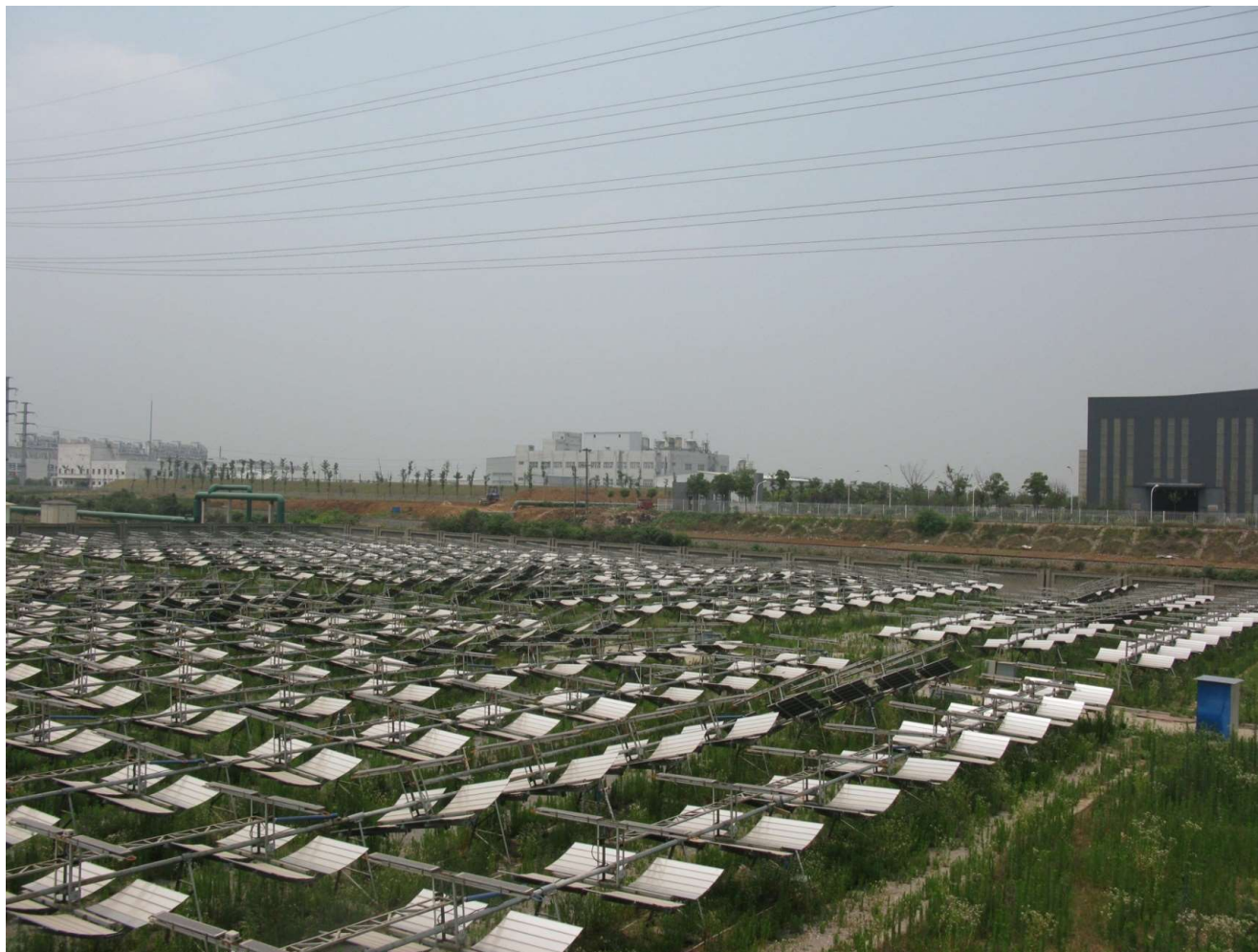
Integrated photovoltaic thermal system (Pukou Base)
